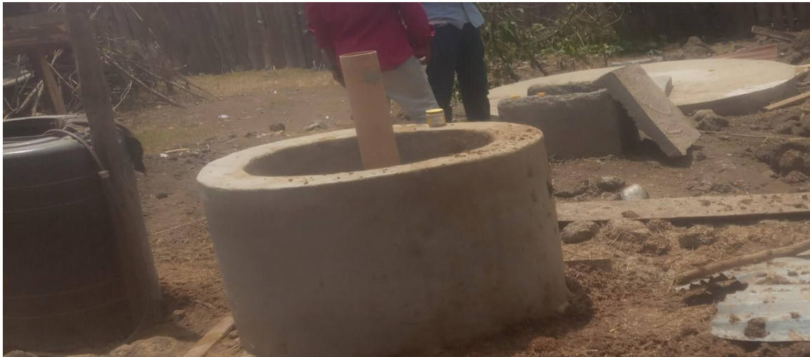
Fixed Dome Bio-Digester
